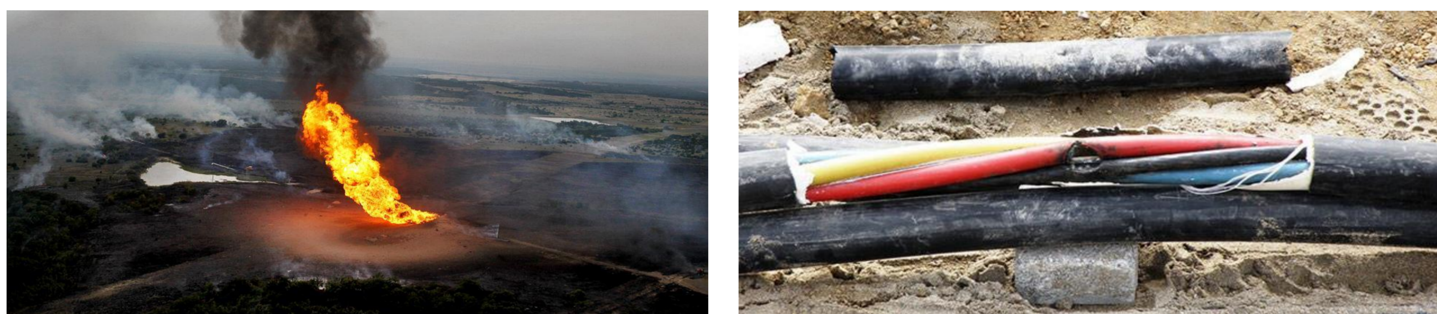
Fig. 1: Application examples - pipeline blast [1] and underground power cable failure [2]
